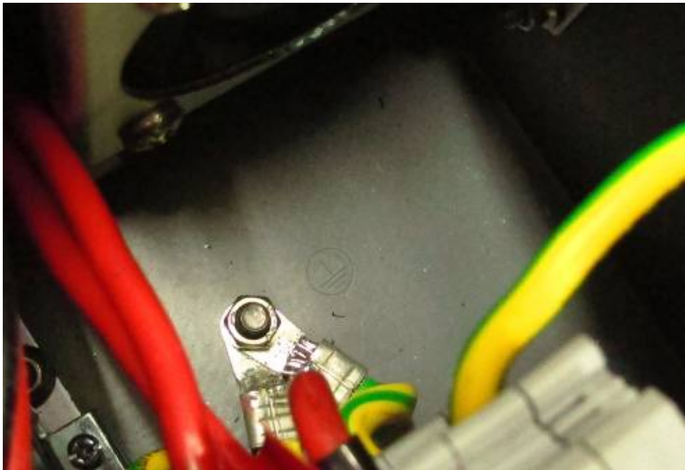
Earthing terminal of the unit
