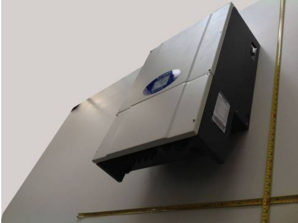
Overall view of the unit
