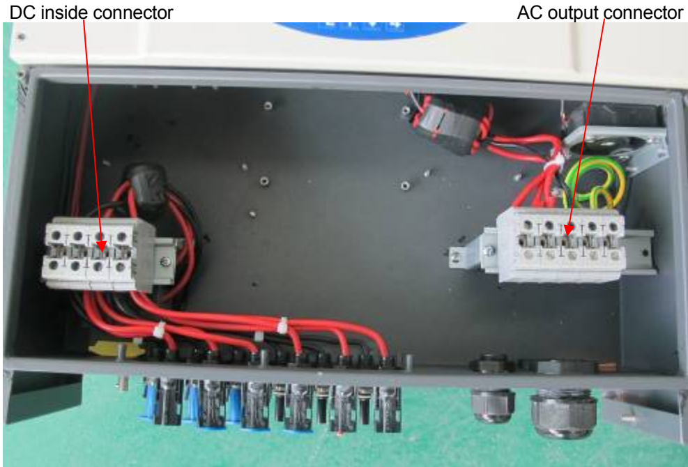
Internal view of the unit
